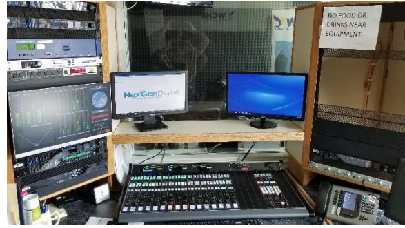
The WCHB control room sporting the new LXE surface.
