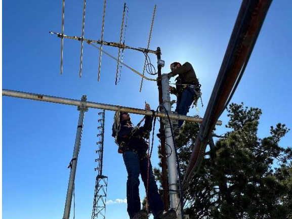
The tower crew works to tighten up hardware on the 95.3 FM antenna at Lookout before raising it to its final elevation.
