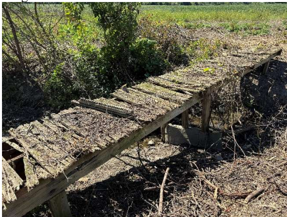
Figure 1 - What was left of the old bridge.
