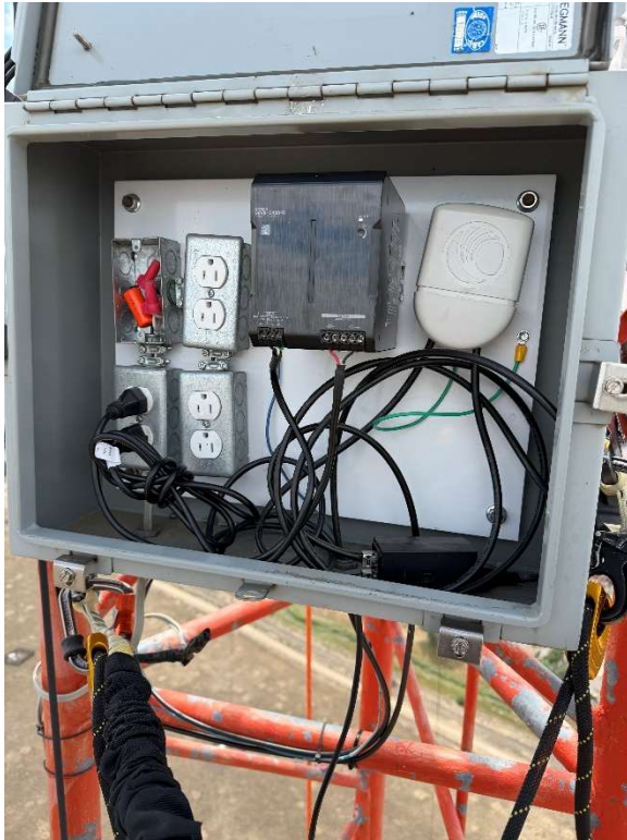
A new Omron 48-volt DIN-rail power supply in place in the NEMA box at the 400-foot level of the KLZ west tower got the link back up and running.
