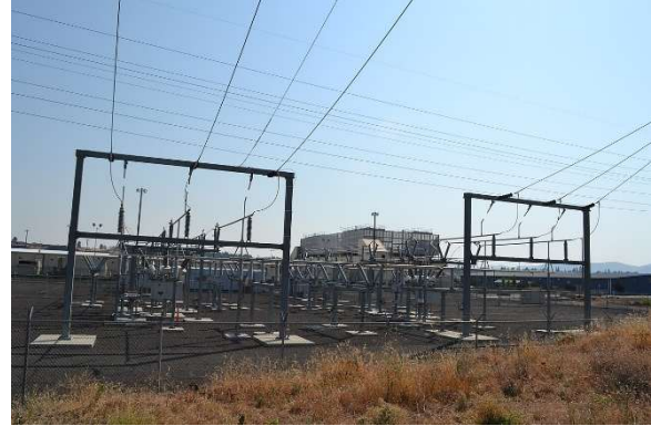
Figure 3 - Power for a Google datacenter in Oregon.
