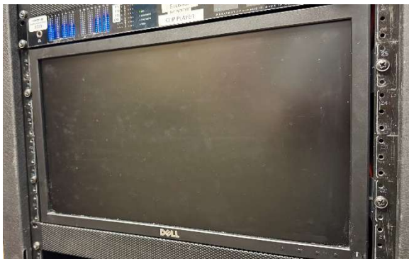
Figure 2 - The fitment of the 19" monitor in the rack (minus some necessary cleaning).
