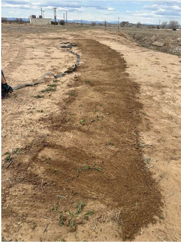
Sixty feet of backfilled trench. I felt every inch. Note the old and damaged strap at the upper right.
