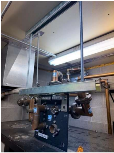
New suspended patch panel.
