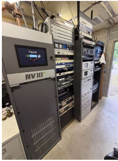
NV10 LT installed!
