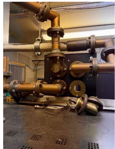
Old transmitter-mounted patch panel.
