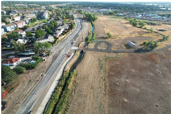
The road widening project at the KLZ site. Our entry is fully restored, but there are still detours in place that make getting there a challenge.
