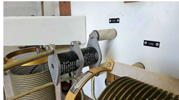
The new capacitor pair in the WRDT tower 2 ATU.
