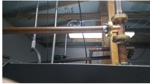
Hard to take a good picture in that small building. The stub is mounted horizontally.
