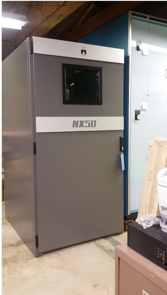
The WMUZ(AM) Nautel NX50 in place next to the Kintronics 10-tower two-pattern phasor.
