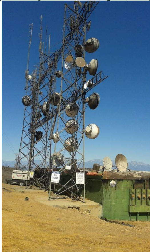
This Sierra Peak roof, several transmission lines/waveguides and antennas were damaged by the Canyon Fire.
